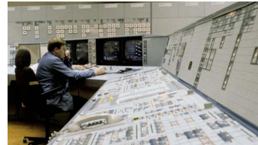
Analogue conventional control room
